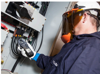
Analyze Power-related Issues
